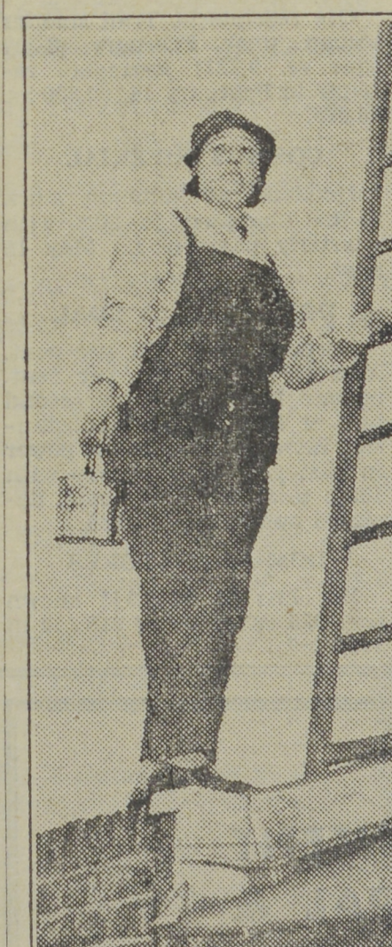
Although she has to look after her three young daughters, MRS. BESIE BURBIDGE finds time to operate a construction business and employ ten men. She is the only woman "working" builder in London, England, and probably in the British Isles. Here we see Mrs. Burbidge about to carry out some repairs on the roof of a house.
