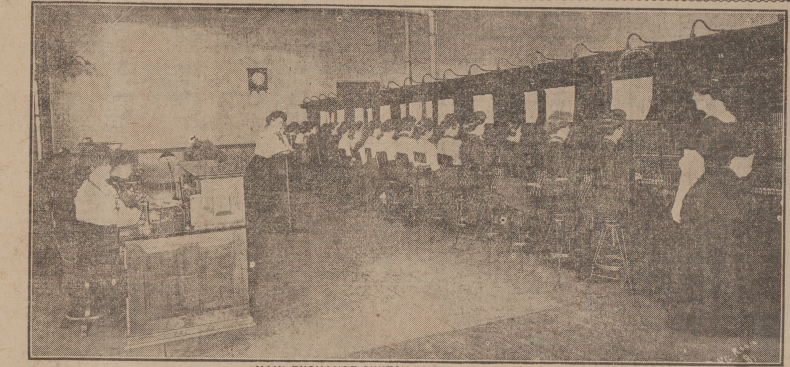
MAIN EXCHANGE SWITCH BOARD, ST. JOHN, N. B.
